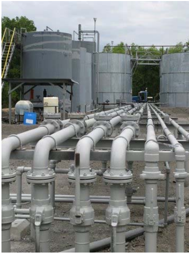
Tank Battery and Flow lines
