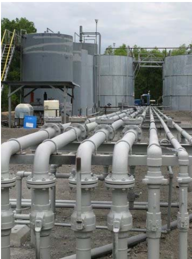
Tank Battery and Flow lines
