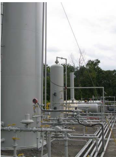
Two and Three Phase separators plus Heater Treator for Jumonville # 1
